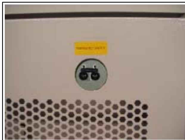
FIGURE 3-3 EMERGENCY BREAKER SWITCH
