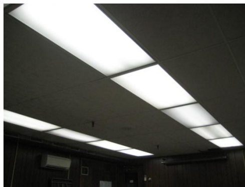
Figure 3: T12 Fluorescent Lighting in Offices, Break Rooms, Bathrooms, and Conference Rooms
