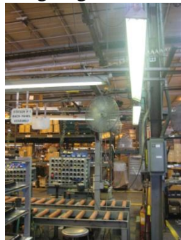
Figure 2: T12 Fluorescent lighting
