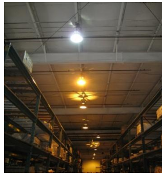
Figure 1: Metal Halide and High Pressure Sodium Lights
