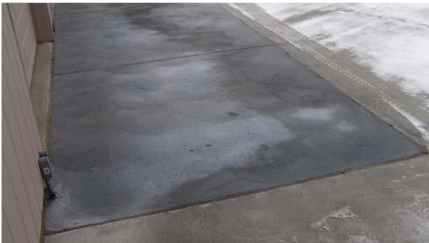
Figure 3: Driveway de-icing – December 2010.
