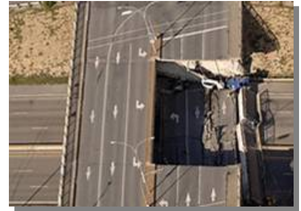
Hwy 19 Overpass Collapse Quebec (2006, 5 dead)
